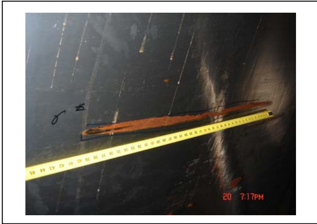
Figure 4.11: A damaged strip showing wedged head
