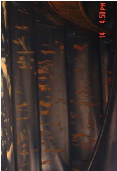
Figure 5 Damages on the lower surface on all guide vanes showing nearly the same pattern
