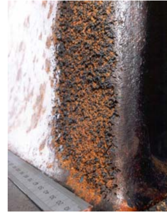
Figure 11 Typical sponge-like erosion pattern caused by a leading-edge cavitation attack (4000 hour operation) [18]
